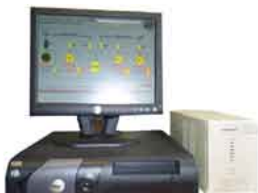
Fig. 8 Control panel based on PC
